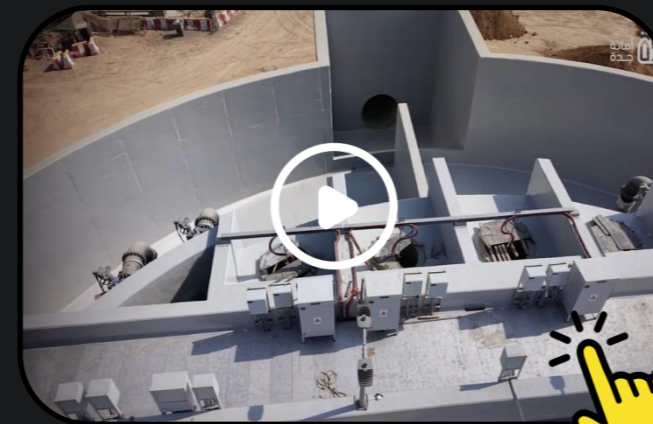
Nahda Water Substation
